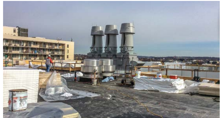
Upblast exhaust fans on roof.
