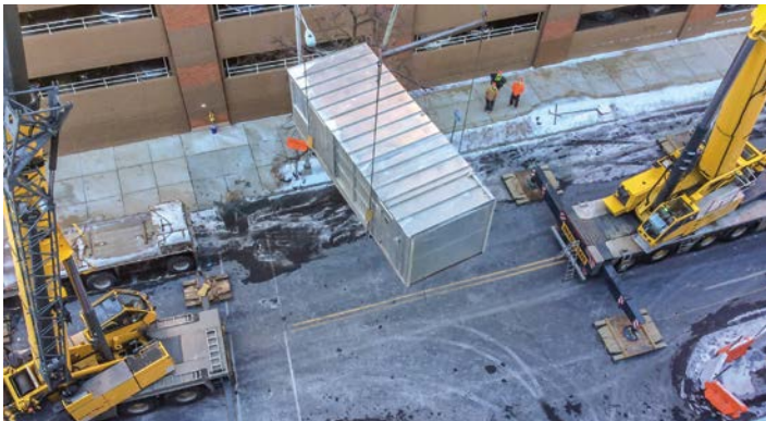
Relocating the air handling unit to the roof required shutting down Chestnut Street in downtown Harrisburg.
