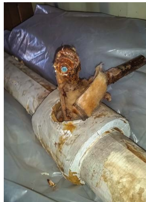
Old, corroded valve.
