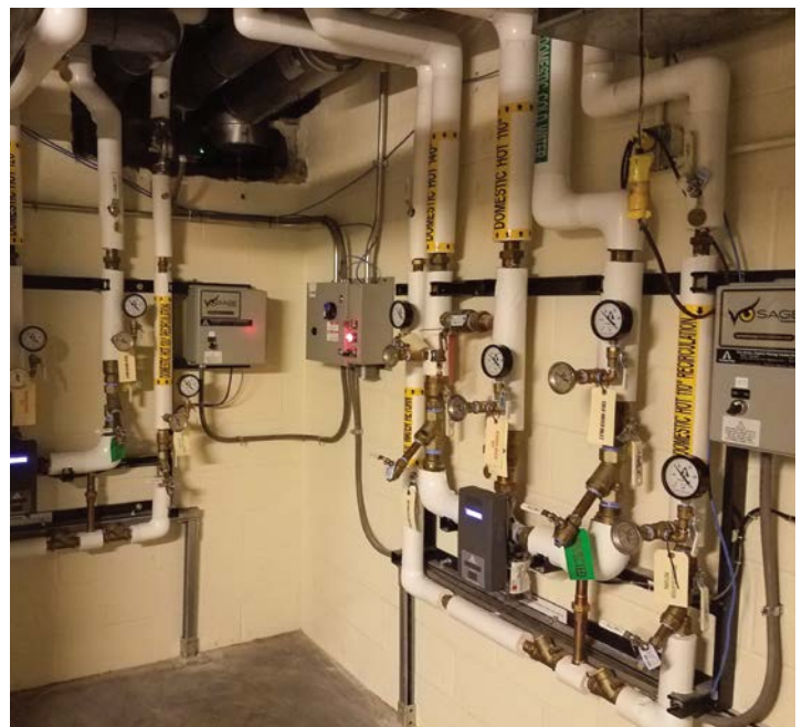
Homestead Village was upgraded with Armstrong digital mixing centers.
