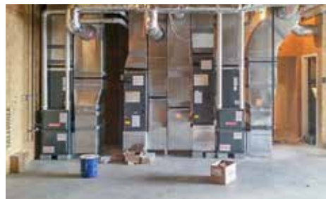
Air handlers and ductwork.
