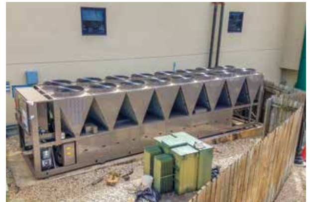
The new chiller in place.
