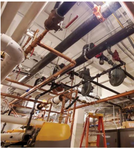
Mechanical room piping and boilers
