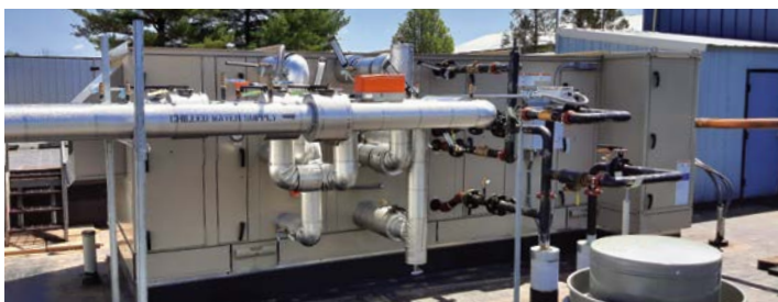
Rooftop Air Handler
