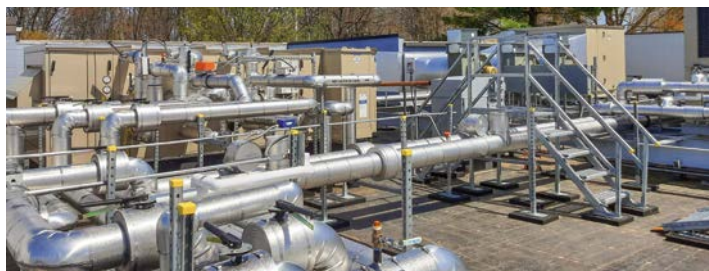
Mechanical Equipment & Piping
